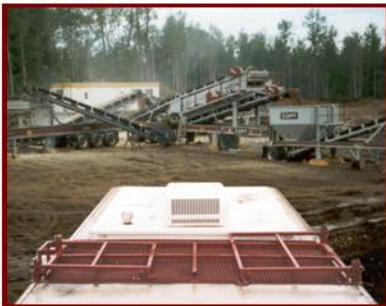
Clemro control towers give you full view of your crushing spread.
